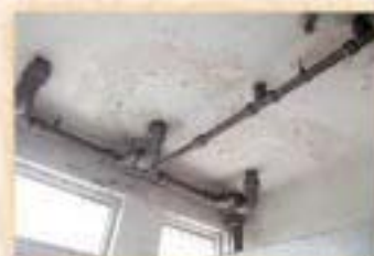
The old walls need repair and the old pipes need replacement
