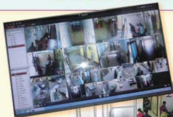
Security and surveillance monitoring system
